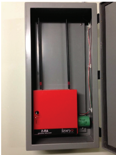
AR-5 Repeater Installed in ES321606-FR2 Enclosure
